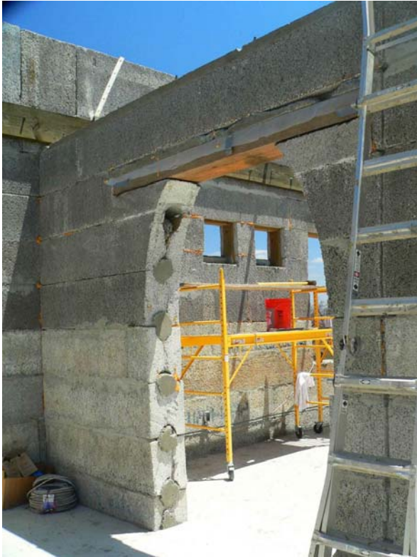
Arches and other covered elements are formed using Perform Wall turned vertically to form a radius.
