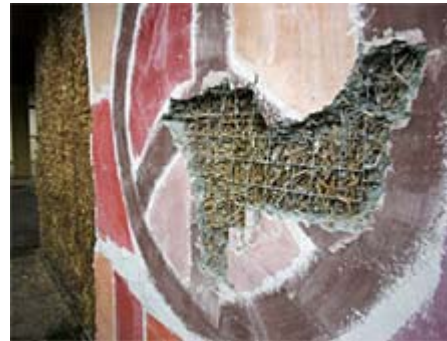
SCOTT LINNETT / Union-Tribune A demonstration wall at the Friends Center tests the durability of layers of stucco, mesh and straw.
